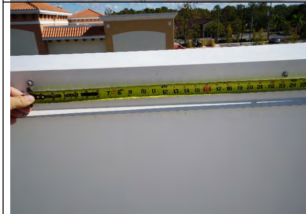
Plans, specifications and contract require coping metal to be secured 12"-inch o.c. This was not in compliance.
