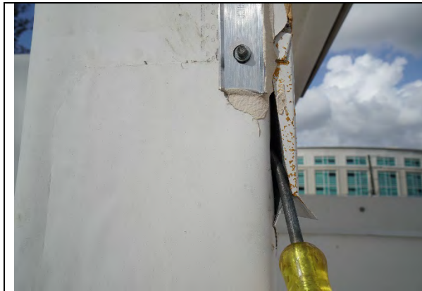
Showing open lap seam underneath counterflashing.
