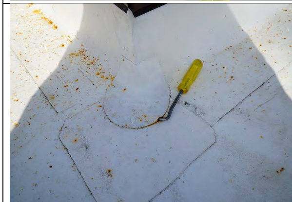
Showing open lap seam at outside corner patch at base of goose neck vent.
