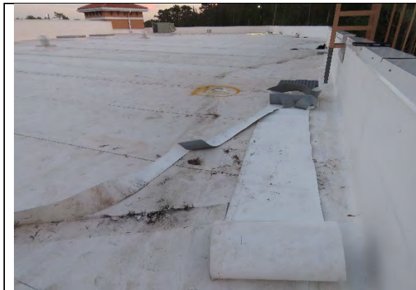
Showing left over TPO membrane left of roof.
