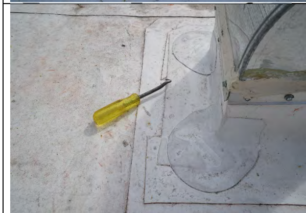
Missing T-patch at base of goose neck per manufacturers requirements.
