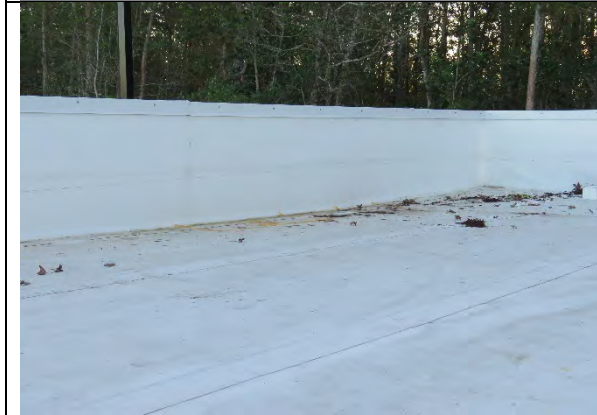
Showing roof deflection at parapet wall/roof connection. This condition allows water to pond. Infrared thermography and capacitance moisture scanner showed elevated levels of moisture. This location is above Quest Diagnostics where active leaks were detected.
