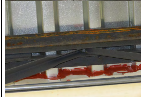
Showing rust on steel trusses under the metal roof deck indicates roof leaks.
